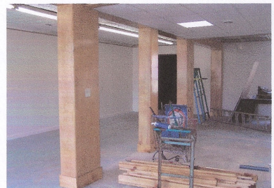
The nearly-completed interior of the front room at the old Hahn & Schaffner store.
